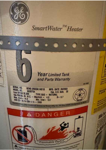
Water Heater Accessible Room 2
