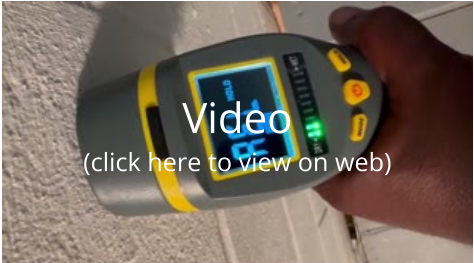
Moisture Detection Upper Wall (Lower Moisture) 2
