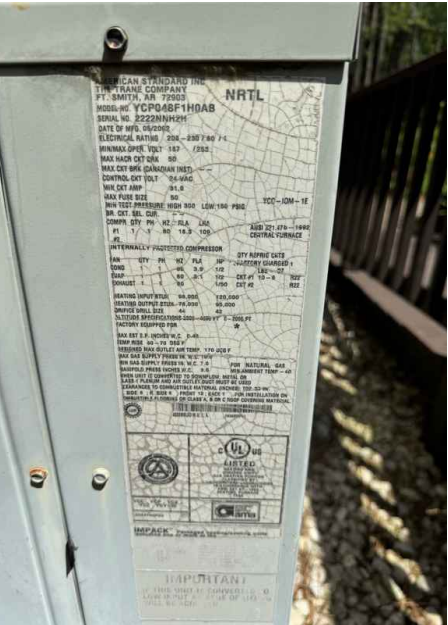
Westside HVAC Package Unit
