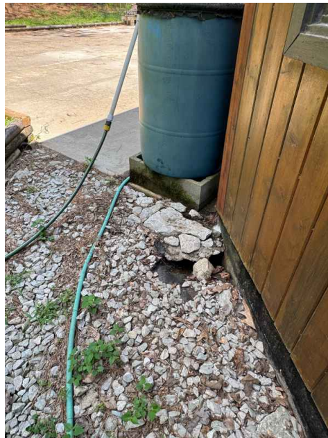
Erosion Hole-Southeast Corner
