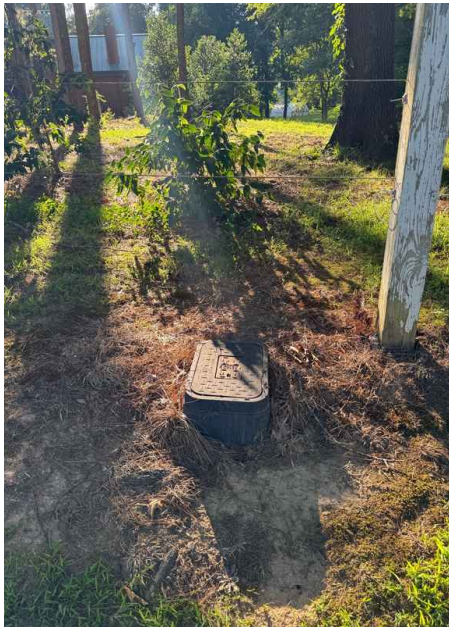
Water Meter Public Roadside
