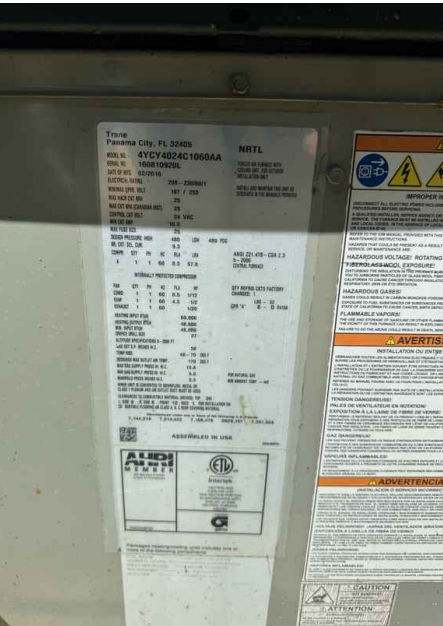
Northside Package HVAC
