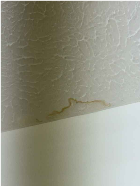
Dry Water Stain 2
