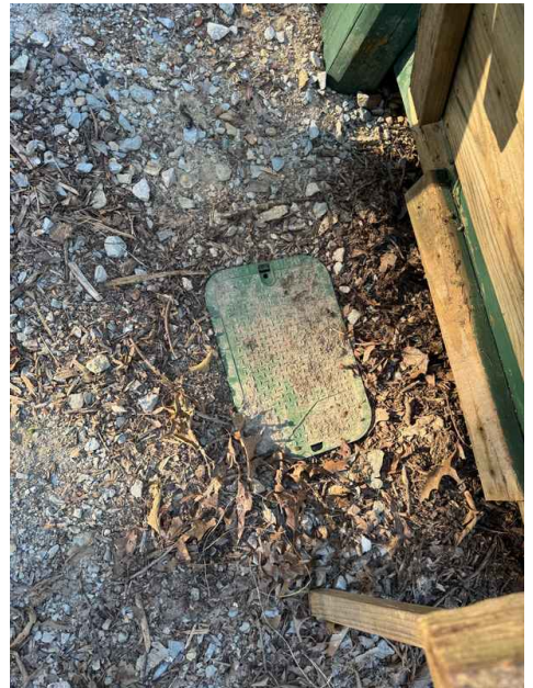
Shut-Off to Workshop
