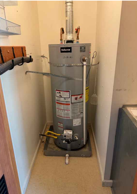
Water Heater Near Great Room
