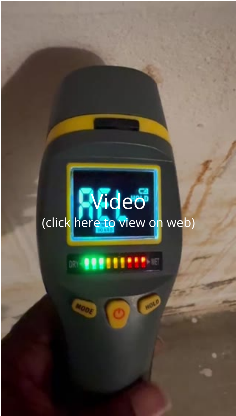
Moisture Detection Lower Wall (High Reading)
