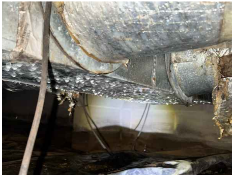
Cooling Ductwork Condensation 3
