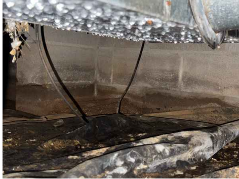
Cooling Trunk Condensation
