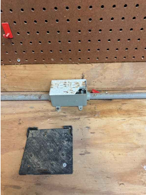
Outlet Cover Damaged
