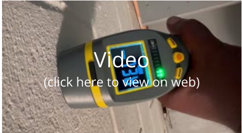
Moisture Detection Upper Wall (Lower Moisture)
