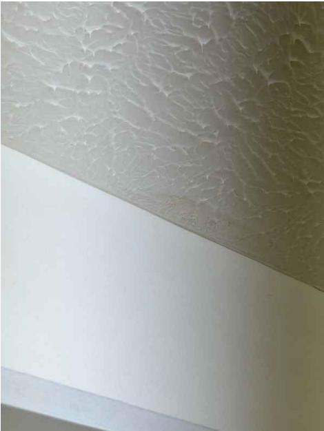
Dry Water Stain
