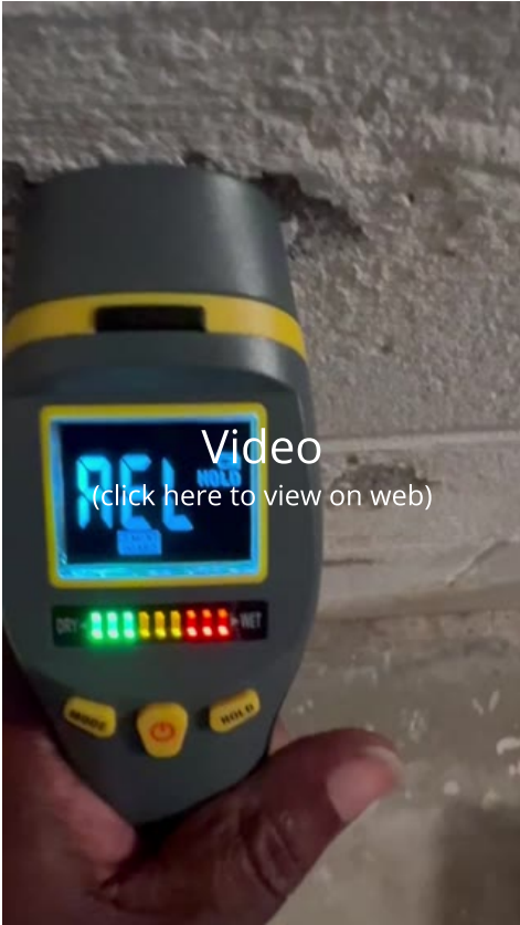
Moisture Detection Lower Wall (High Reading) 2
