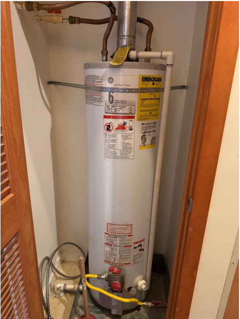
Water Heater Accessible Room
