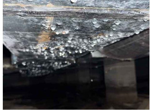
Cooling Trunk Condensation 2
